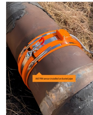
MsT probe for permanent monitoring installed on a pipe
