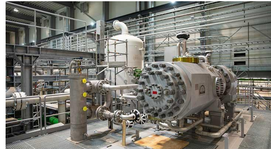
MAN Heat Pump Unit
