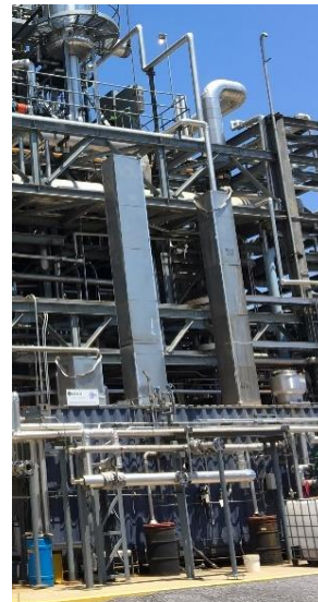
Pilot Testing at SSTU, NCCC (2018)
