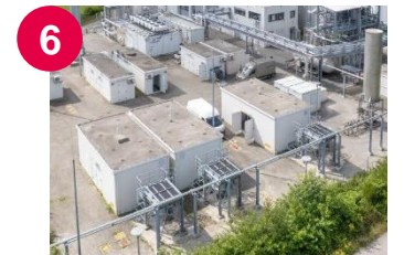
CH4 feeding into gas grid
