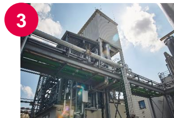
Methanation reactor system
